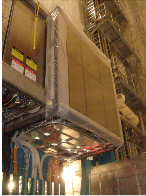
Figure 2.12: View of the installed POD from beneath. [48]
