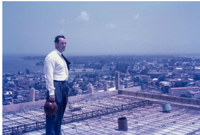
Figure 149:1961 picture of Charles C. Stevenson on the roof of Independence House under construction 527
