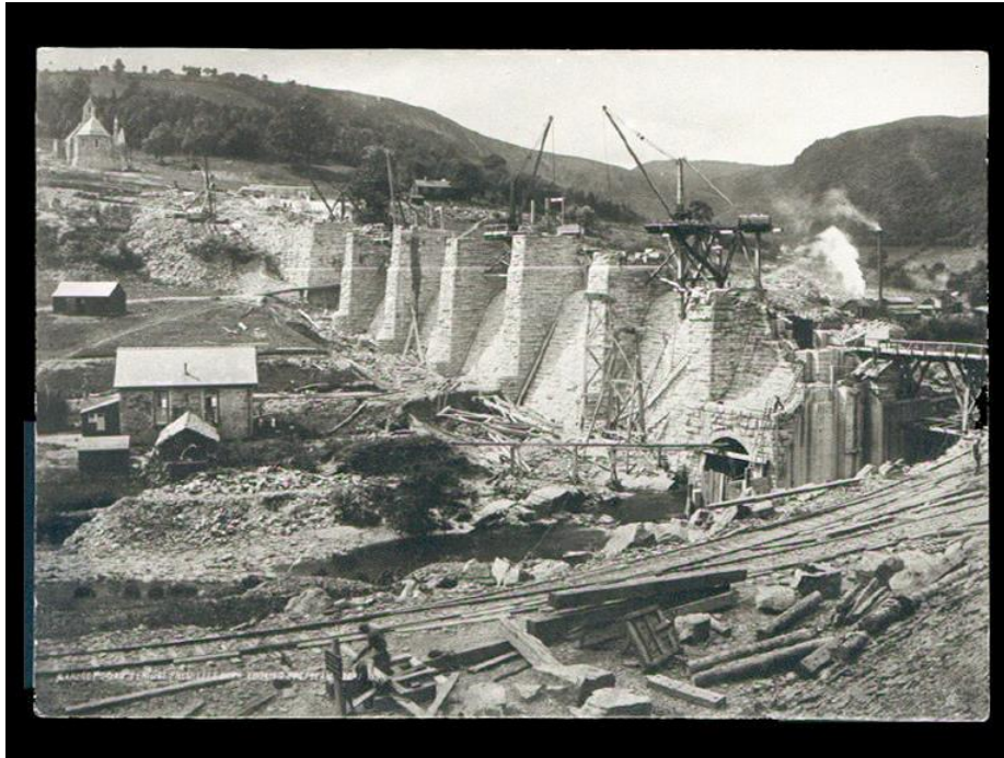
Figure 7: Construction of the Elan Valley dam (This image appears in Betty's digital story. It was provided courtesy of BBC Wales. Date and copyright unknown)
