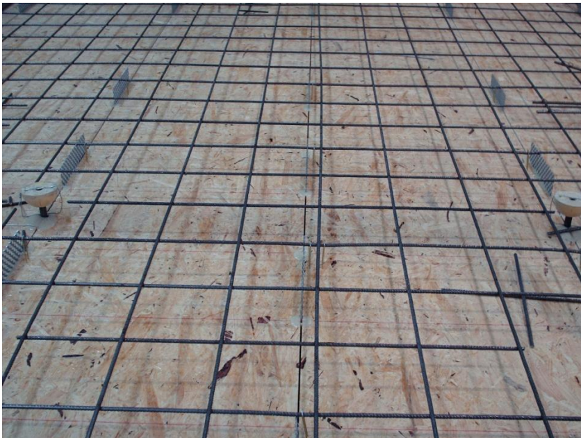
Figure 2. Lines of shear connecting strips protruding through the OSB before the concrete is cast on a nominally identical floor (NB This photo also shows the steel reinforcement mesh.).
