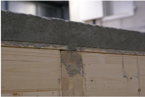
Figure 3. Timber joist in contact with the concrete.
