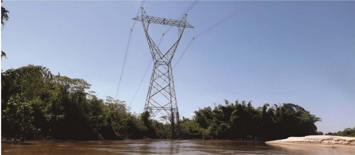
Fig. 21. Energy transmission network that needed to be relocated owing to the intense channel changes in reach 1.
