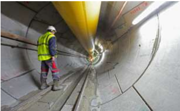
(a) INELFE tunnel between Spain and France
