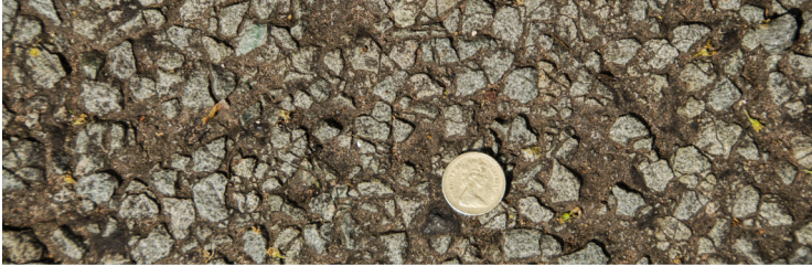
Figure 5 Photograph showing a worn road surface with aggregate raised above the bitumen matrix. £1 coin for scale. (photograph M. Williams)
