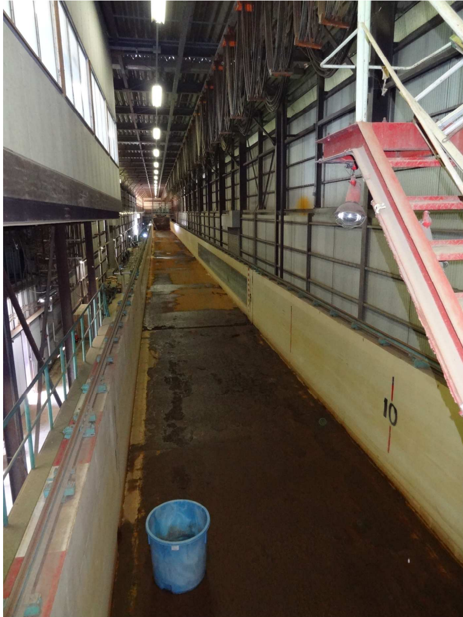
bed of flume looking downflume showing rusting flume bed
