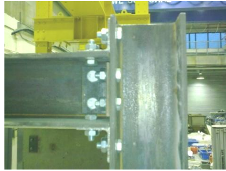
(b) Beam-column connection on the right hand side of the second storey
