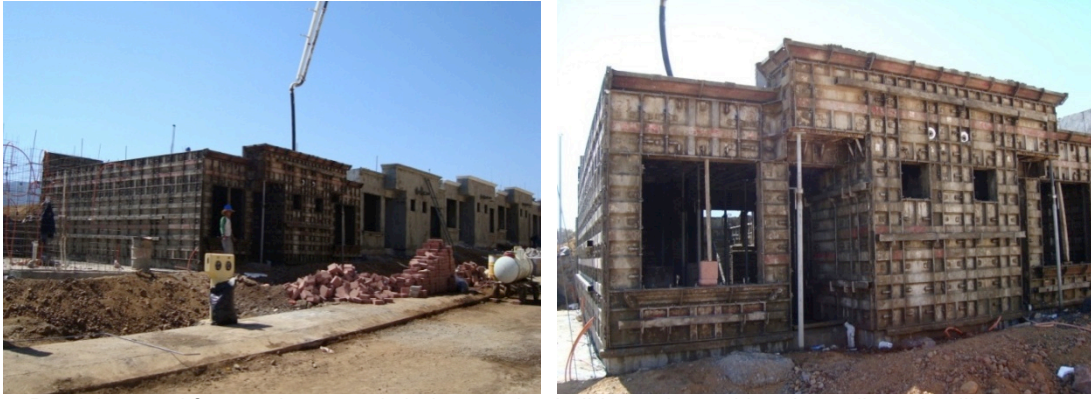
Fig. 3. Precision steel formwork system is being used to build exterior and interior walls and ceilings at one time.
