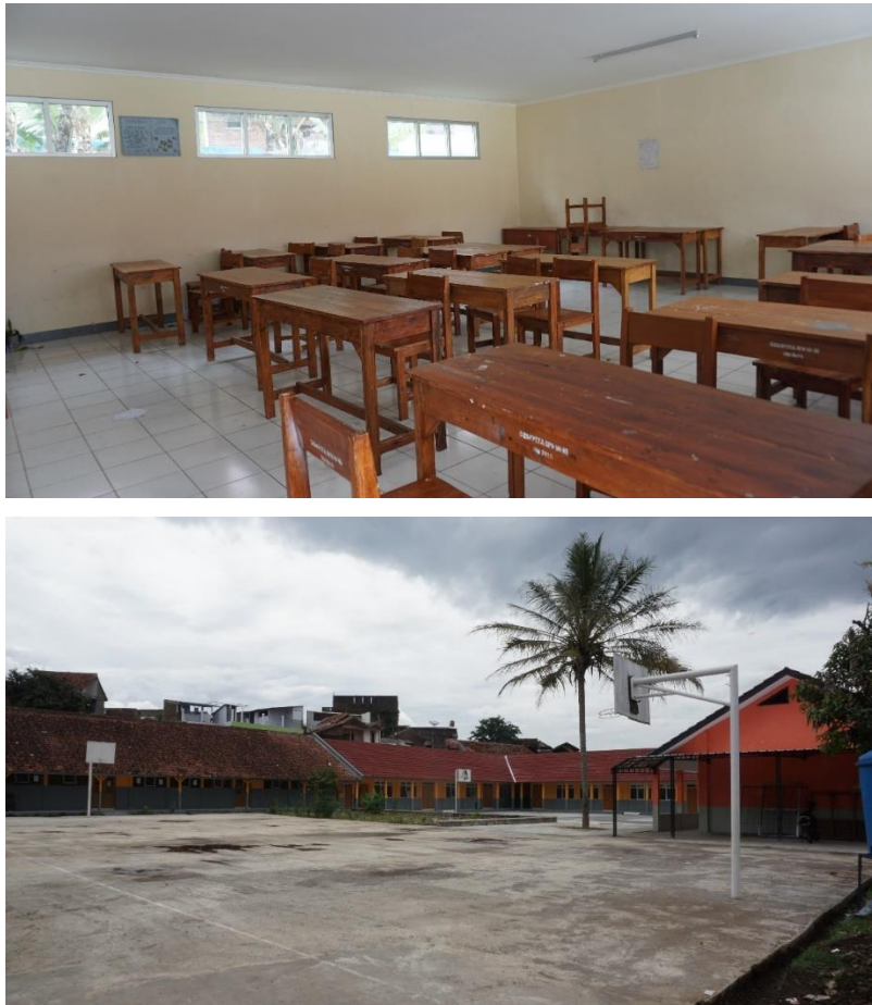
Figure 22: All classrooms in one of schools facing repeated flooding do not have evacuation exit doors and alarm installed (top image). There is no evacuation sign in school yard (bottom image).
