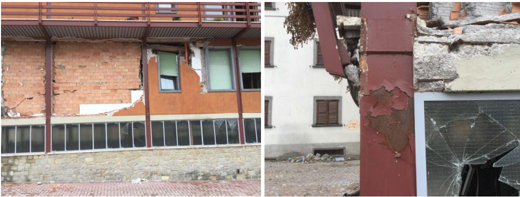
Figure 3. Surveyed damage of the case study building after the 2016-2017 earthquake sequence (significant damage on infills and yielding at beam-column connections).
