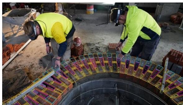
Fig. 6: AR 3D instruction for complex wall assembly. This figure was produced by Fologram in 2020 [56], and it summarized that the unskilled labors are assembling the complex brick wall guided by the AR 3D virtual holographic instruction through Microsoft HoloLens 1. The permission to re-use the figure has been granted by the author and the publisher.
