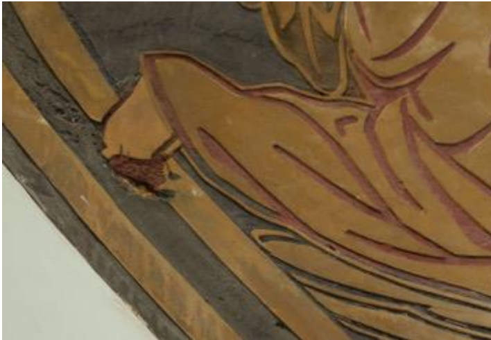
Fig. 9: Delamination of top plaster coat.
