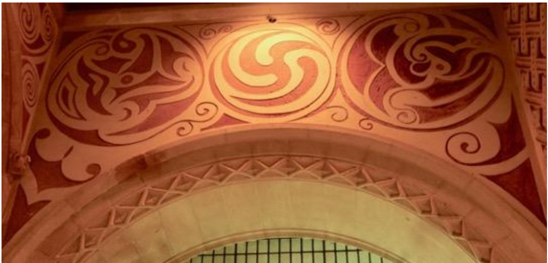
Fig. 7: Sgraffito patterning over the south transept arch, which also occurs on the chancel arch to the left. This view reveals damage to the colour coat from scraping away the topcoat especially in the right hand circle.
