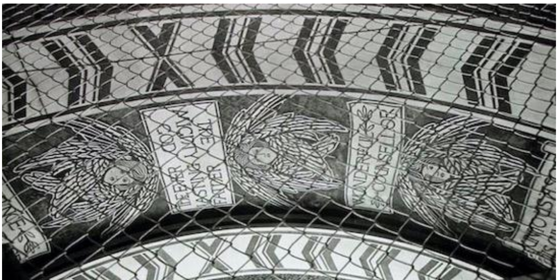
Fig. 13: Lady Chapel, centre of soffit to chancel arch. Angels' heads within wings.
