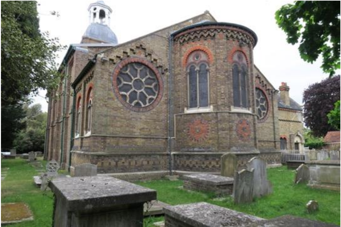
Fig. 3: East end, showing Teulon's apse and side chapel extensions with polychromatic brick details.
