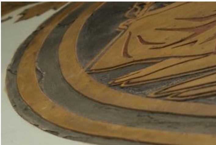
Fig. 10: Salt damage and decay of colour coat of plaster.
