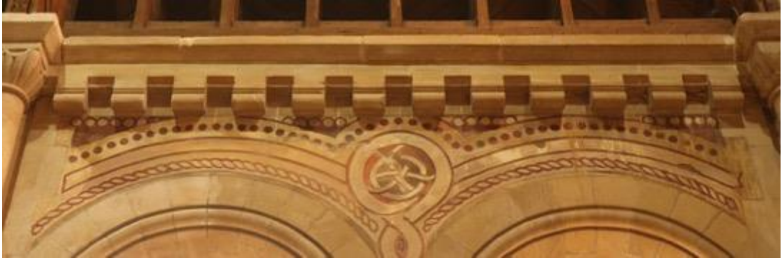
Fig. 5: Sgraffito over the south chancel windows, with what appears to be a variation on a Chi Rho symbol for the name of Christ.
