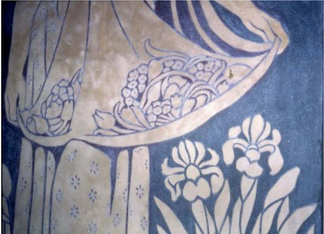
Fig. 10: Detail of Flora, showing the top coat to be a lot thinner than that used at St Mary's five years earlier.
