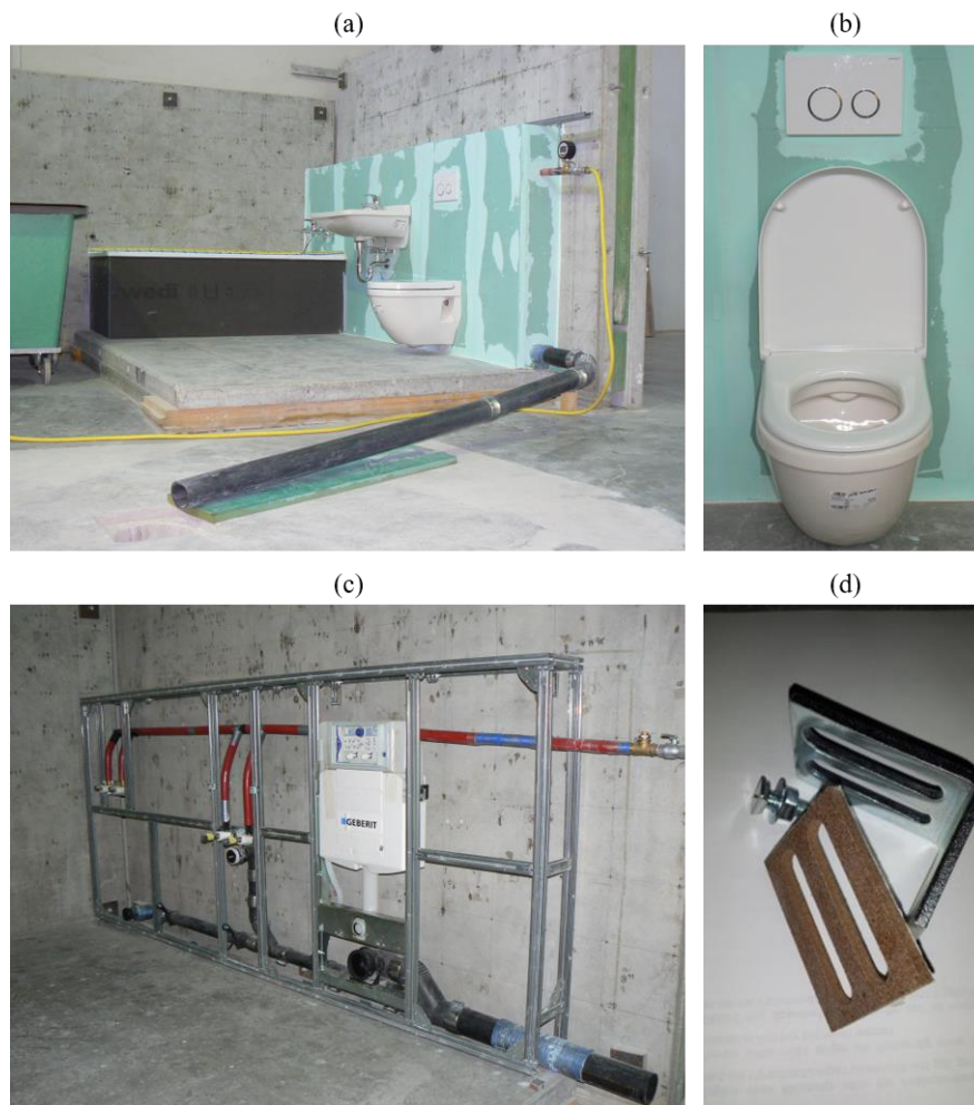
Figure 8-1. Case study of a toilet flush: (a) measurement set-up for the pre-wall installation system (Geberit GIS) with sanitary equipment, (b) the toilet, (c) the load-bearing frame including the installations of the cistern and the fresh- and wastewater pipes and (d) cork layered brackets which fix the frame to the reception plate test rig [37]. This sanitary installation system is installed without the installation shaft for the fresh- and wastewater supply.
