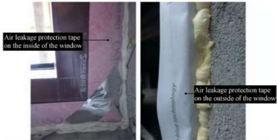
Figure 4-5: Air leakage protection membrane used on both inside (left) and outside (right) of the window in a Passivhaus in Hunan, China.
