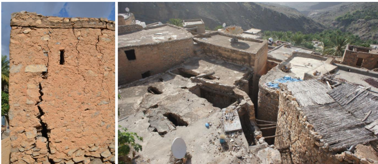
Figure 20: Plaster cracks on the walls because of water infiltration (left) and collapsed roofs due to a combination of rain and lack of maintenance (right) (Bandyopadhyay et al., 2015:70-121).
