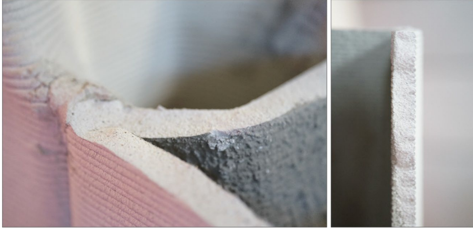
Figure 31: A closer look at the cracks
