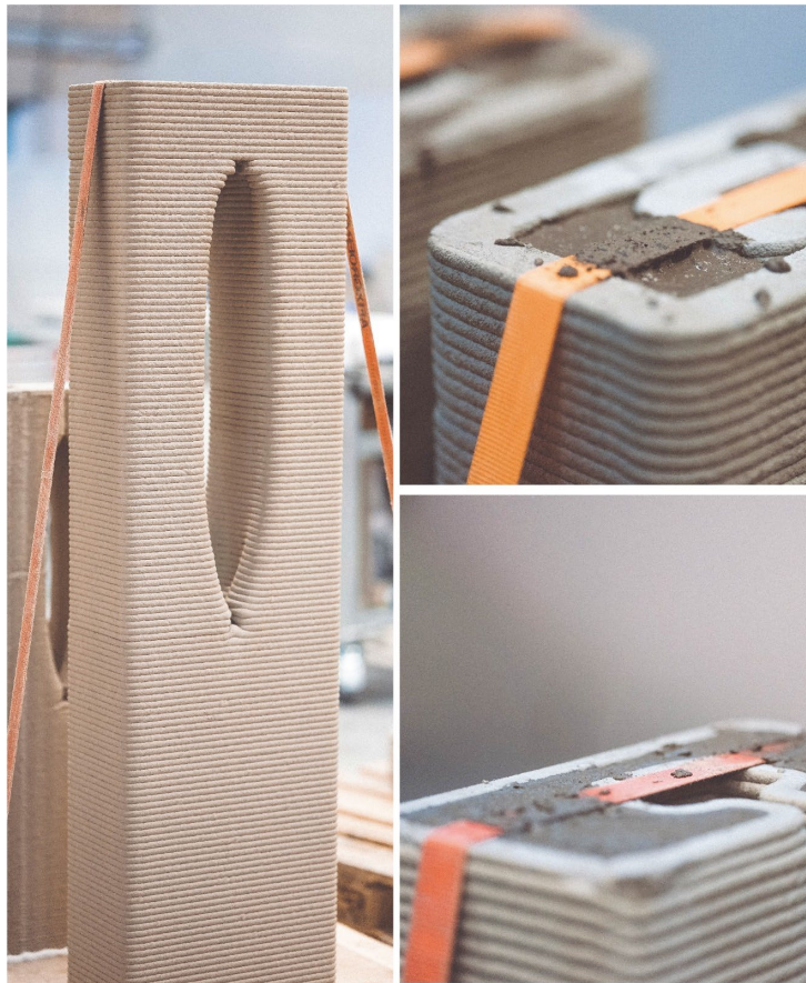
Figure 25: Securing the prints with straps to prevent potential hydrostatic pressure between printed layers when the concrete was poured
