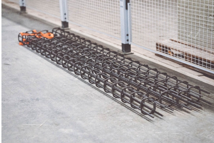
Figure 23: Reinforcing the full-scale column with rebar 4 cages; each cage has 12 mm longitudinal bars
