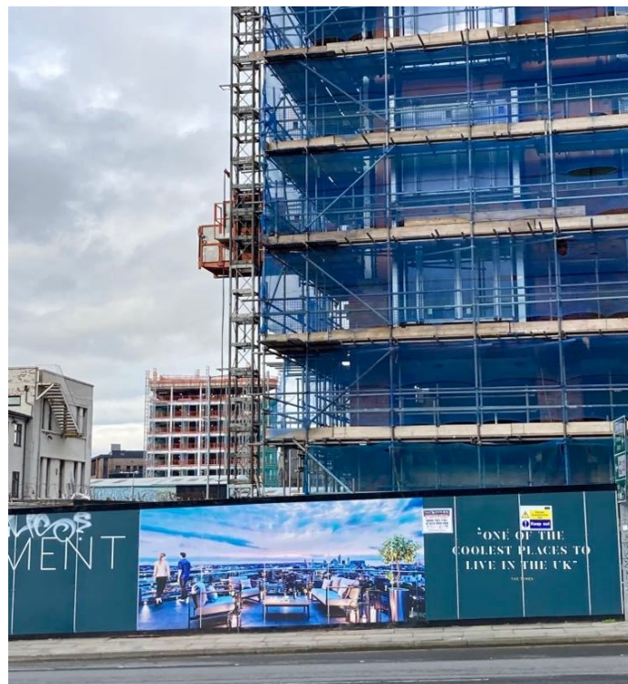
Figure 4.10 “The coolest place to live in the UK”, work-in-progress residential development in the Baltic Triangle
