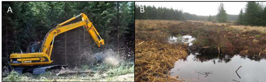
Figure 1.7. A) A digger mulches timber in the Long Grain catchment © Tony Bartholomew. B) Long Grain after forest clearance and ditch-blocking © Forestry Commission.
