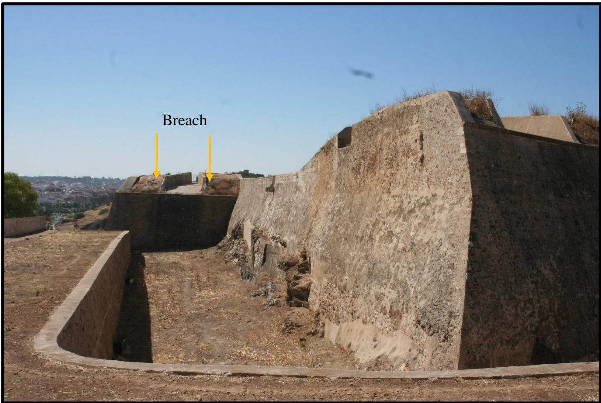
Figure 6. Location of the San Christóbal breach made during the second siege. (Photograph taken by the author July 2017).
