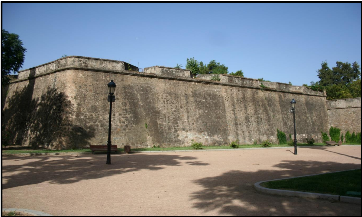
Figure 20. Left flank of the Santa Maria bastion. The breach was located between the two lamp posts shown in the picture. (Photograph was taken by the author August 2015).
