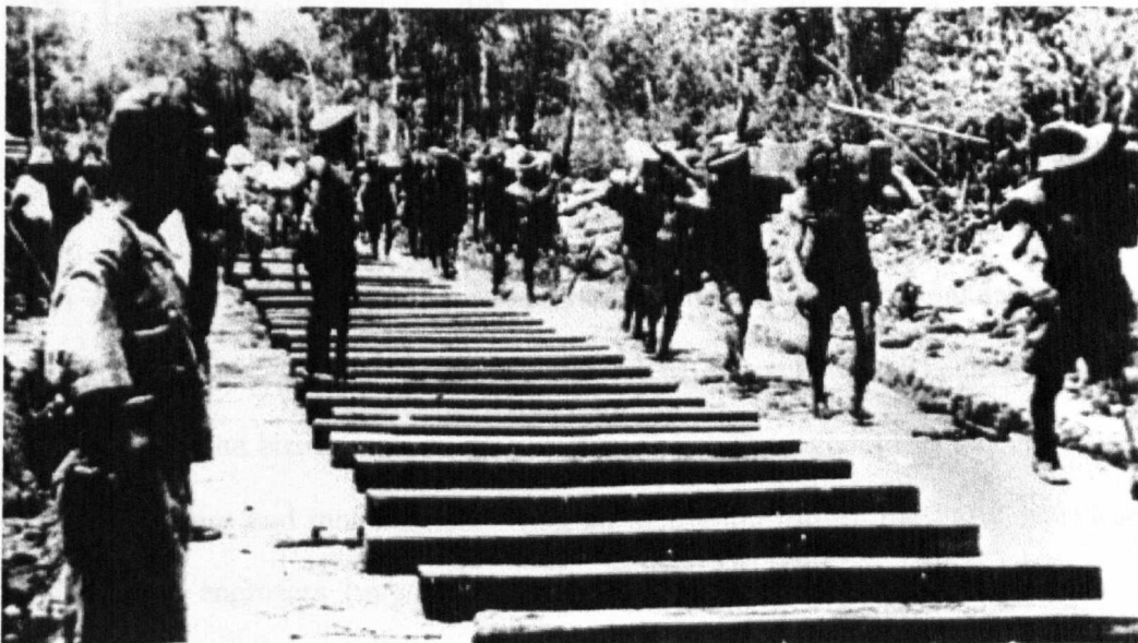
Figure 5. Building the railway. An Australian POW group of "line carriers" about to place a line on the previously laid wooden sleepers (contemporary – and probably secret – photograph from the collection of Brigadier Philip Toosey, courtesy of Professor Peter Davies).
