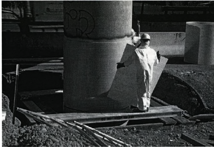
Figure 1.8. Reinforcement of concrete column with FRP composites to improve strength and seismic resistance [28].
