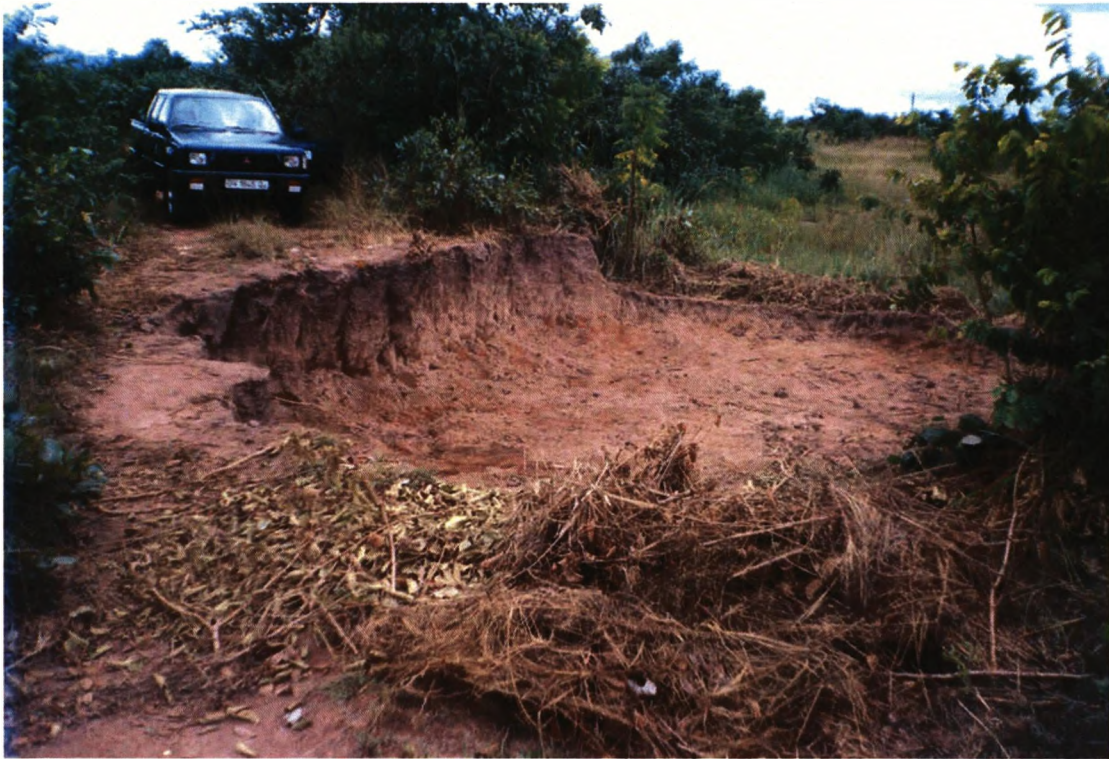
Vital rural and farm road made impassable as a result of stone and sand digging activities
