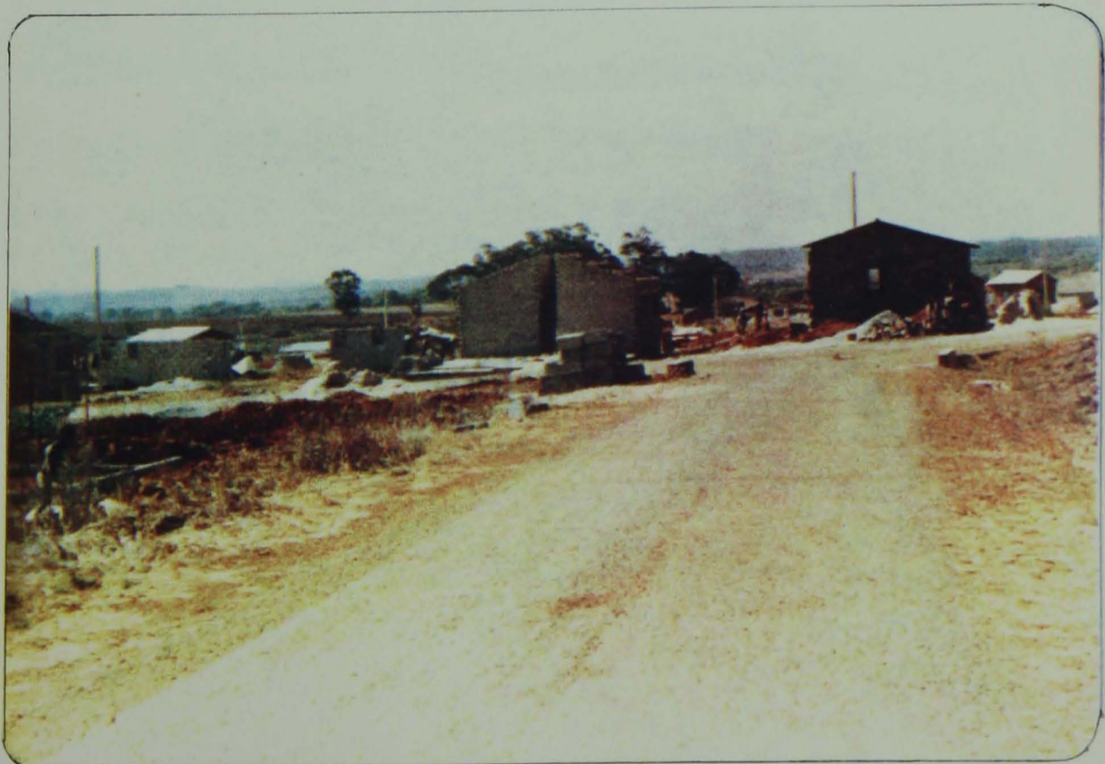
Plate 6.3a - Another view of Hatcliffe housing estate showing the already tarred road and the high level of construction in progress.
