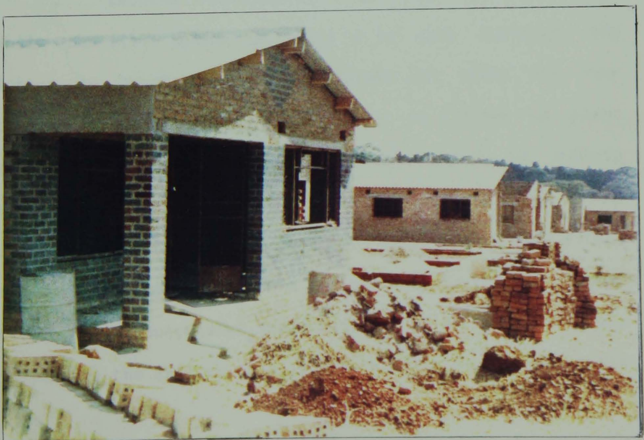
Plate 5.4 - To a well built solid house. Note construction in progress in the background.
