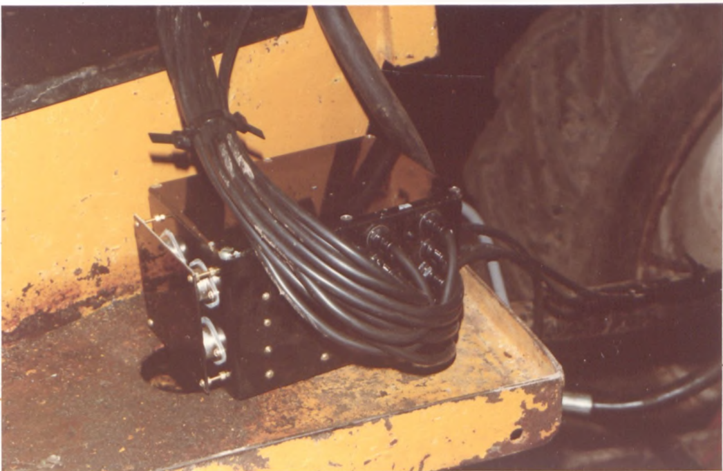
Plate XIV: Power Switching Unit
