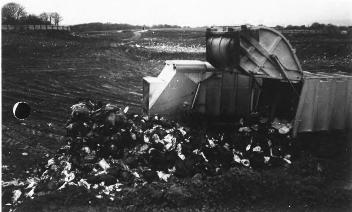
Plate 4. Etna Landfill Site, Alyn and Deeside: Located in a former Clay Pit.
