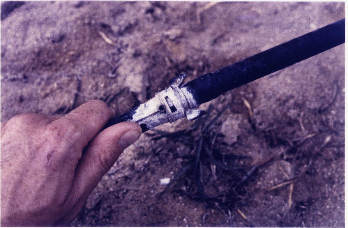
Plate 5.6 Calcium carbonate precipitation on the surface of a Type A Emitter supplied with potable water (emitter discharge efficiency is unaffected)
