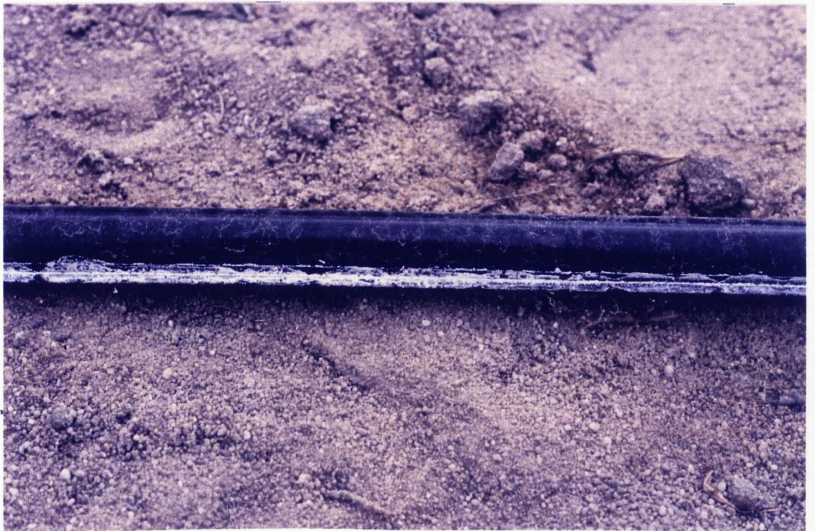
Plate 5.7 Calcium carbonate precipitation on the surface of a "Seephose" lateral supplied with potable water
