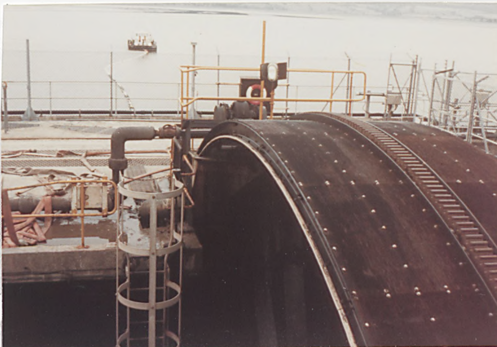
Plate 2.13, Oldbury Power Station, Severn estuary, the large revolving drum can be seen in the foreground. In the background the edge of the reservoir can just be seen.
