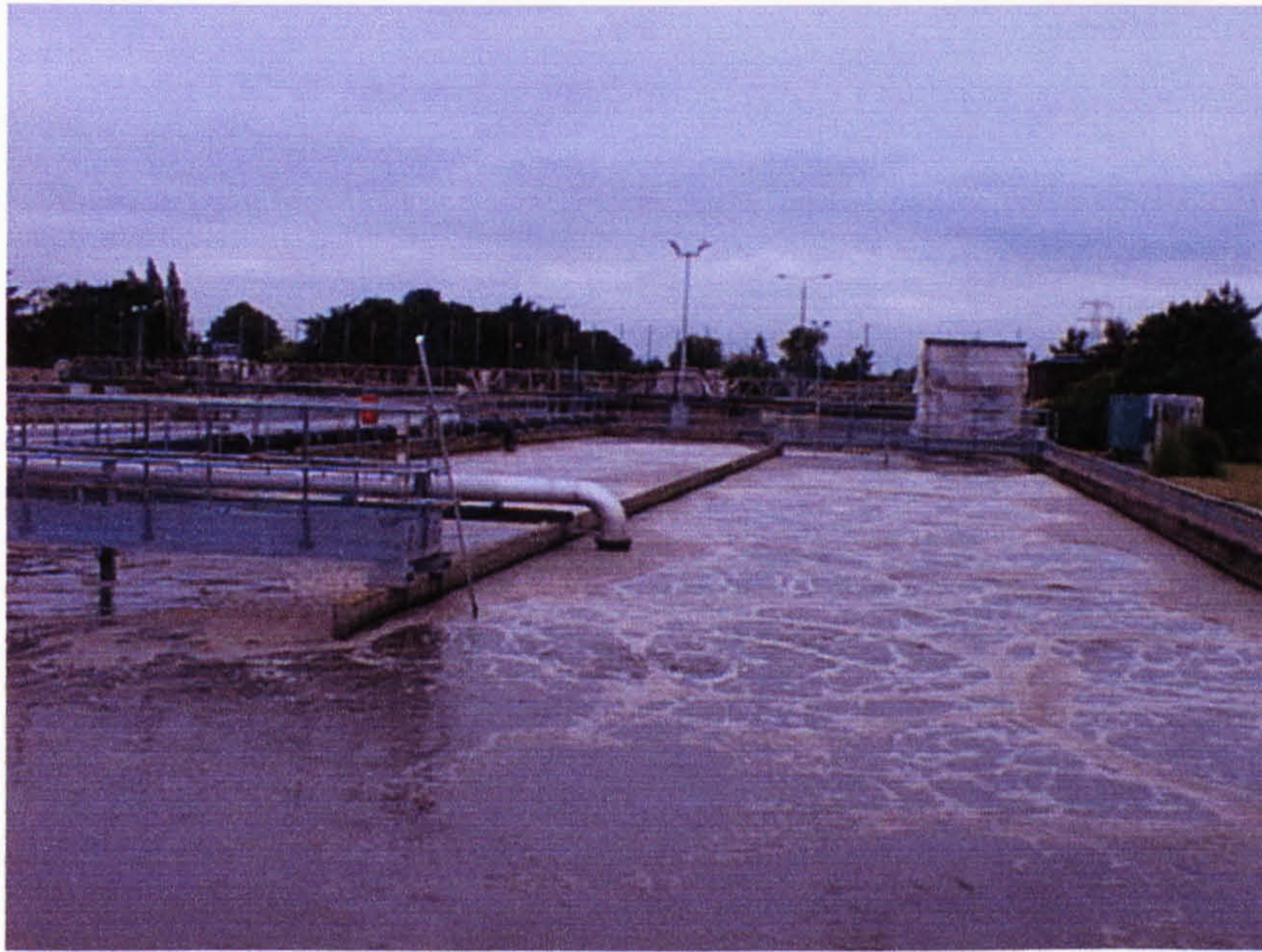
Figure 3.1. Primary settling tanks at Exeter treatment plant from which raw sludge was obtained
