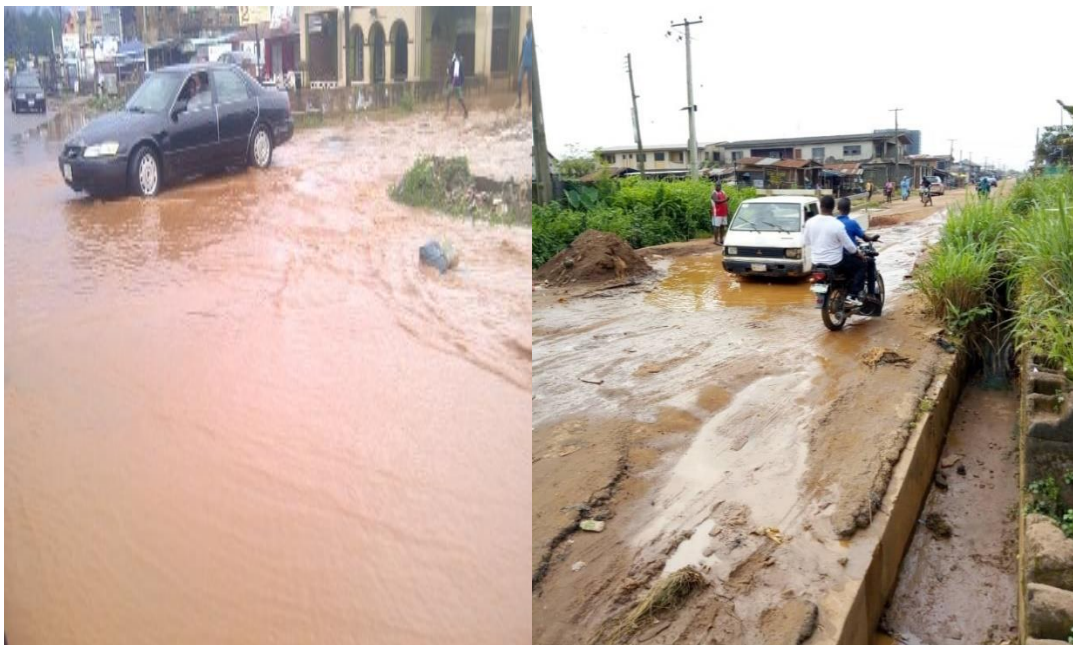
Figure 1.3: a) clogged drain and flooded road; b) silted drain with growing plants and its impact on roads in Ijebu-Ode.
