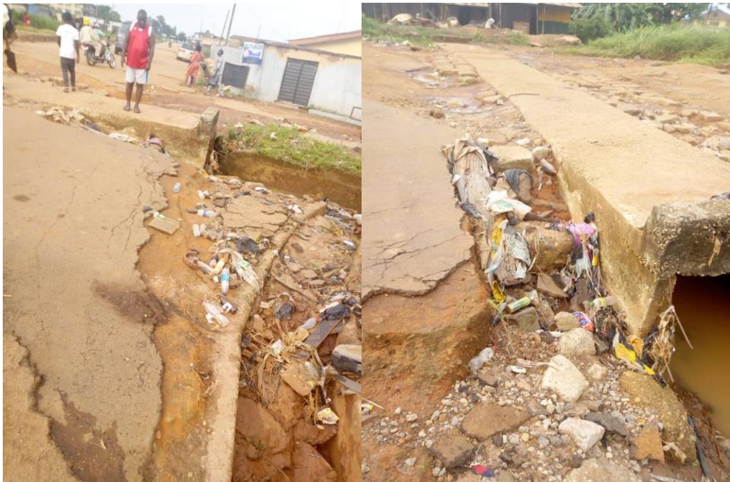
Figure 1.7: a) & b) impact of poor drainage systems and flood on roads asphalt in Ijebu-Ode.
