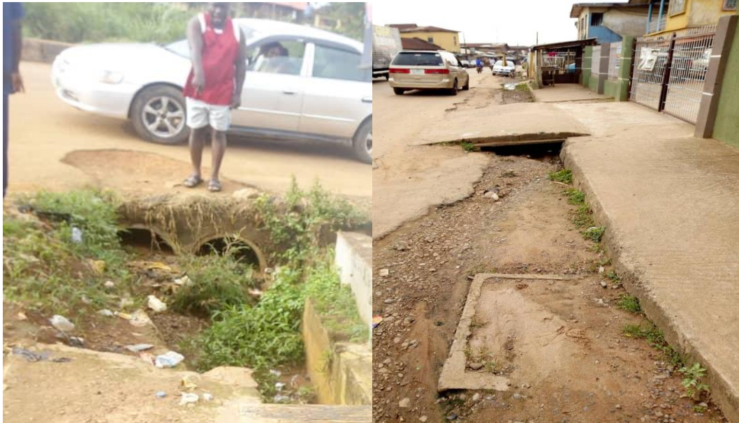
Figure 1.4: a) blocked small old concrete ring drain; b) completely silted-up drain that crisscross Ijebu-Ode
