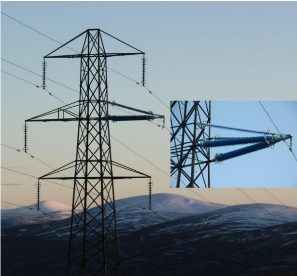
Figure 5 Insulation cross-arm installed on a redundant line in Scotland for two years' load testing.
