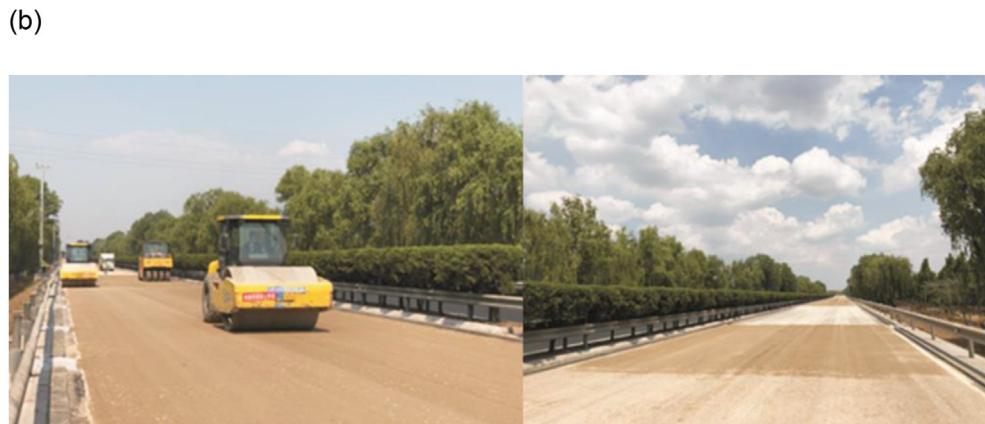
Fig. 48. Comparison and application. (a) Comparison of conventional and inverted pavement structure. (b) Application of high quality unbound aggregate base in Taian, Shandong Province.
